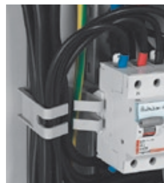
^ The enclosures have wiring guide rings
