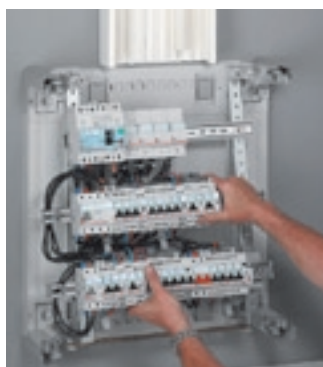
^ When the side panels have been removed, the wiring is fully accessible
