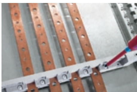
^ Flat bars at the back of the enclosure
